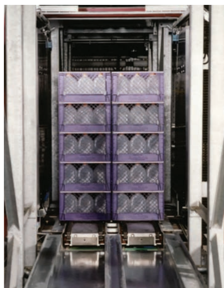
Palletless Dairy Case Stacks transported on Satellite rack entry vehicle within an AS/RS
