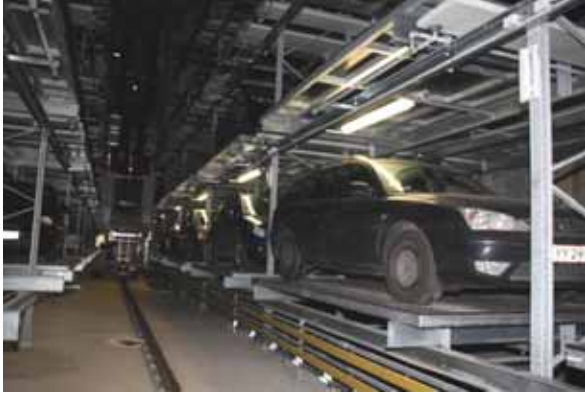
Below ground: Insight into Copenhagen's second fully-automated parking garage in Leifsgade.
