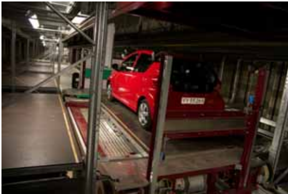
Below ground: Insight into Copenhagen's first fully-automated parking garage at Nørre Allé.
